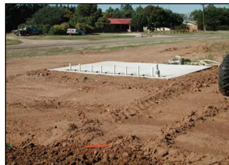
Figure 5. Concrete base for SDI water filter and zone valve control station, TAES, 2005.
