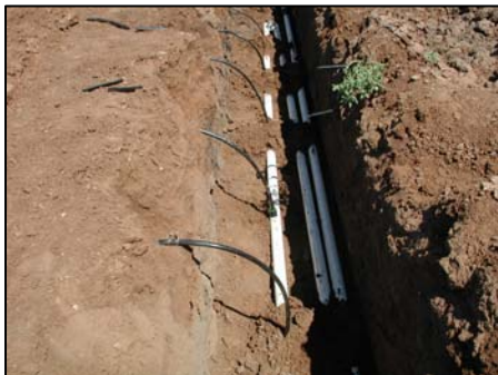
Figure 4. SDI drip lateral connection to water supply manifolds, TAES, 2005.
