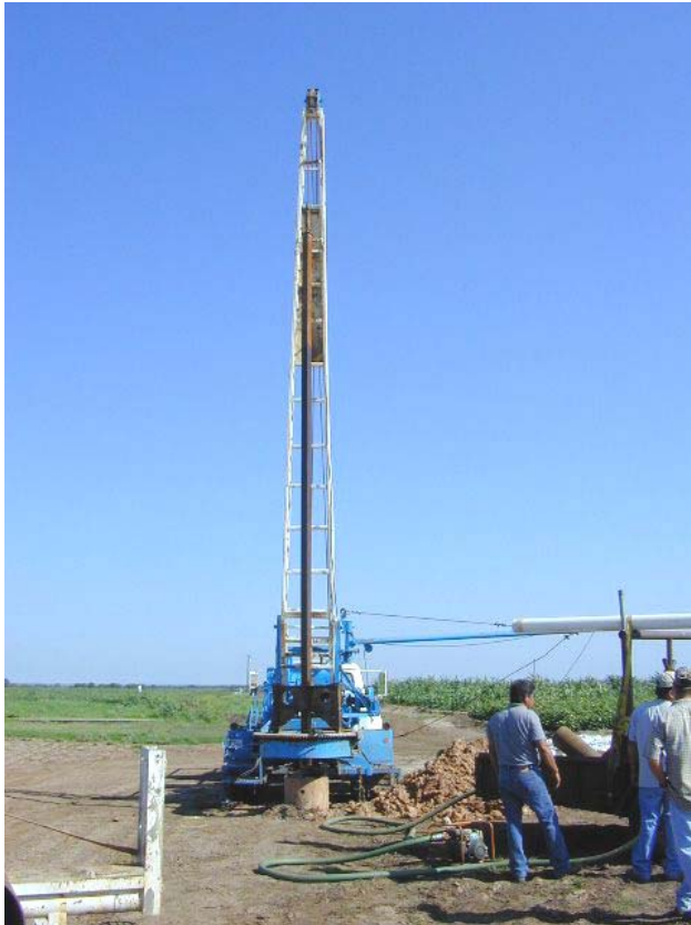
This water well was installed at the Chillicothe Research Station during the summer of 2005.
