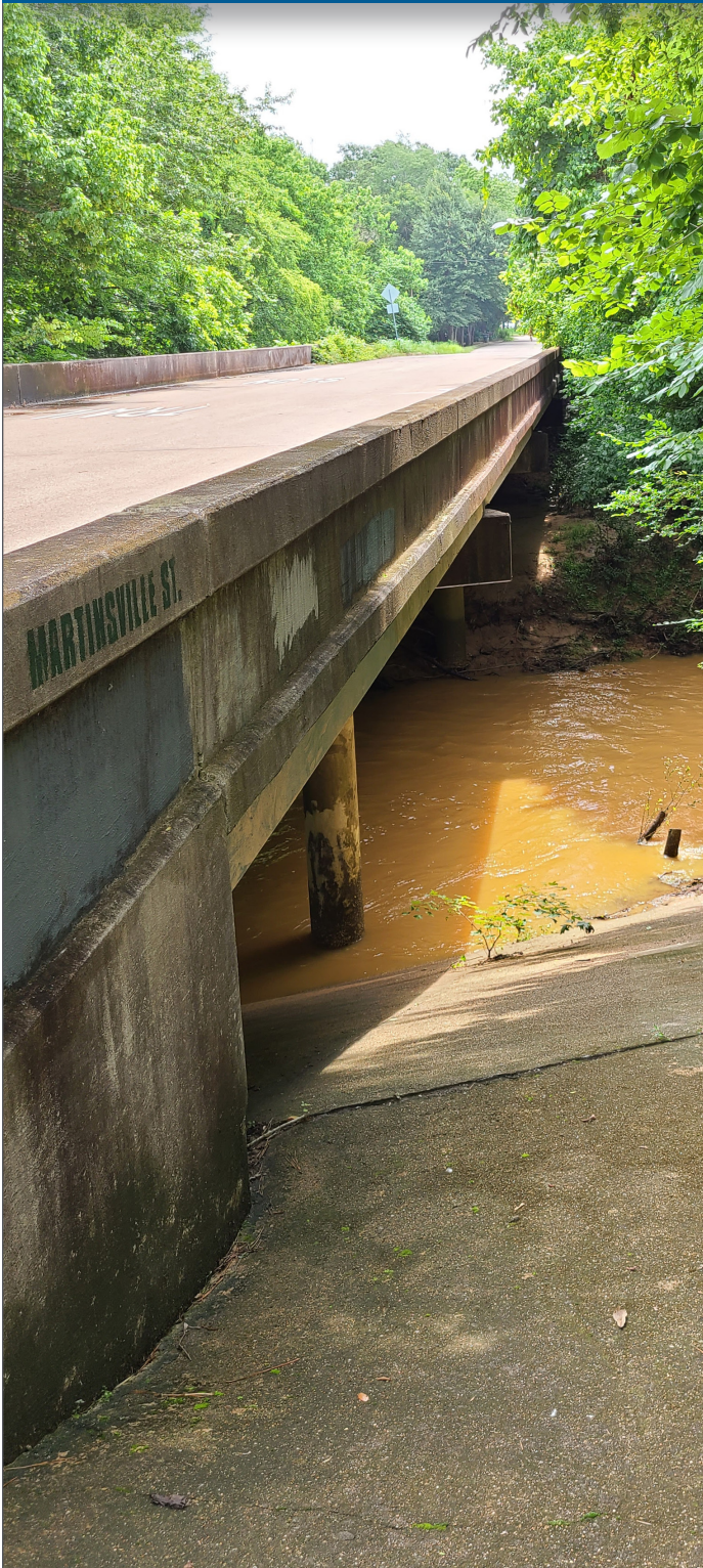
La Nana Bayou bridge crossing at Martinsville St. Photo by Emily Monroe, TWRI.
