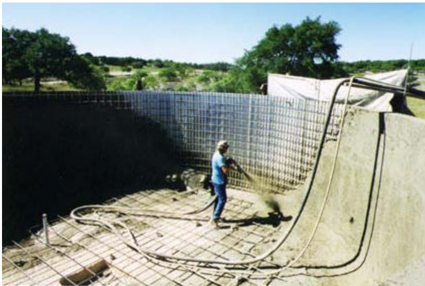
A proprietary concrete is sprayed monolithically over re-bar to form the inside of the main cistern at Avera Armadillo Acres.
