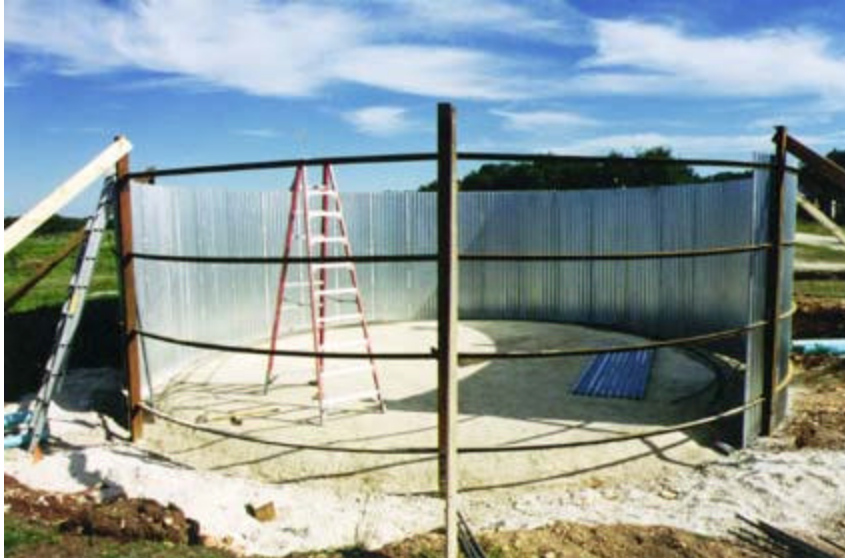
To construct this 40,000-gallon tank at Avera Armadillo Acres, Sustainable Homesteads first bolted together a frame, then mounted galvanized steel panels to the frame.
