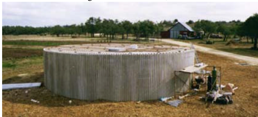
The centerpiece of the rainwater collection system Avera Armadillo Acres in dripping springs is this 40,000-gallon site-built concrete tank. This photo shows reinforcing steel in place before the concrete roof is poured. The rainwater harvesting system at the organic farm was engineered and constructed by Sustainable Homesteads of Wimberley.
