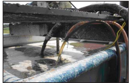
Fig. 3: Mixing tank with chemical additions
