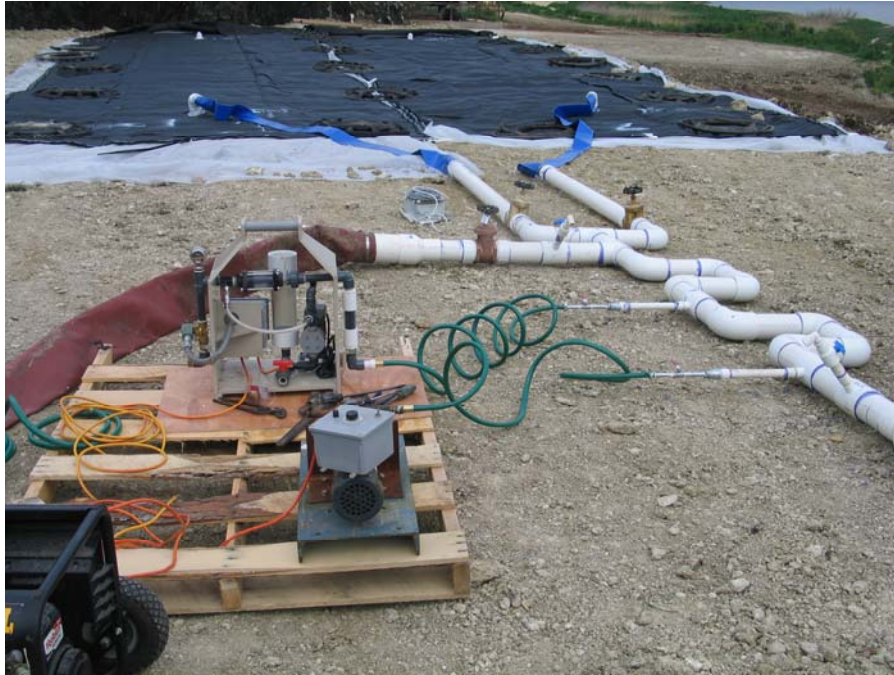
Figure 2. Pump and chemical metering system to mix chemicals into lagoon effluent being pumped in to Geotubes.
