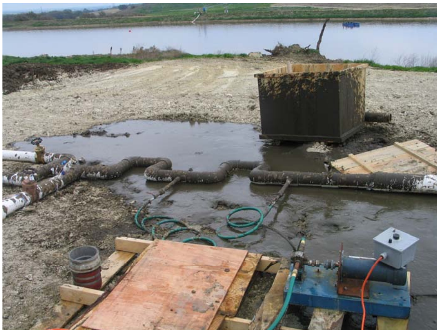
Figure 3. Waste material drenched on monitoring equipment from unclamped hose.
