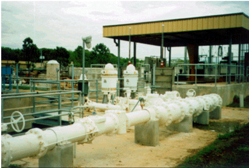
This is the pump station and ozone treatment facility used by the Clear Lake City Water Authority to disinfect reclaimed wastewater for reuse.
