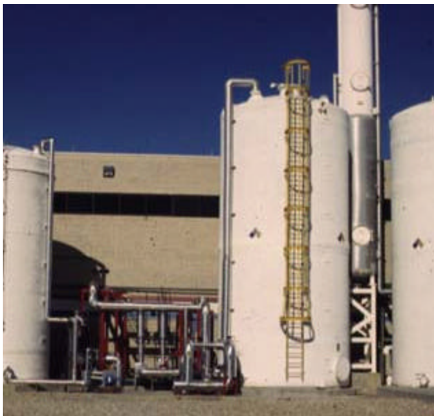
For storing reclaimed reverse-osmosis water, this 20,000-gallon storage tank represents the largest expenditure in SEMATECH's water reclamation project.
