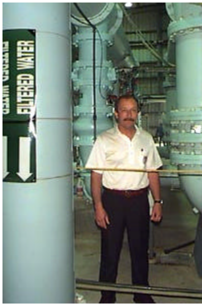
Don Roach of Patricio MWD inside a new microfiltration plant which will supply treated wastewater to a steam electric power generation plant.
