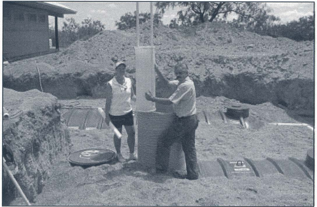
Susan Parten and Louis Hamilton of SEPCO install this septic tank and effluent filter at the Lake Colorado City State Park.
