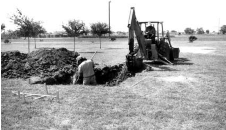
Workers excavate this area where a microbial rock plant filter will be installed.
