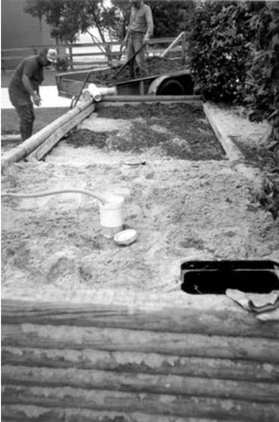
Some homeowners near Lake Livingston are converting existing drainfields to drip irrigation systems like this one (above) because of space and soil constraints.
