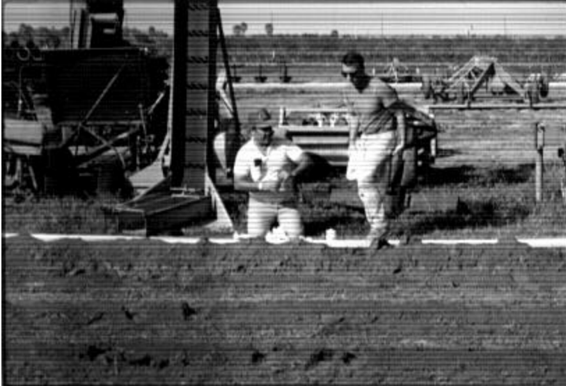
This drip irrigation field is being installed in Weslaco as part of an integrated system that includes constructed wetlands.
