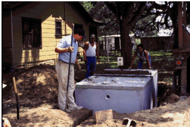
Bruce Lesikar (standing) helps install this septic tank in D'Hannis. The septic tank will work with a constructed wetlands to treat household water.
