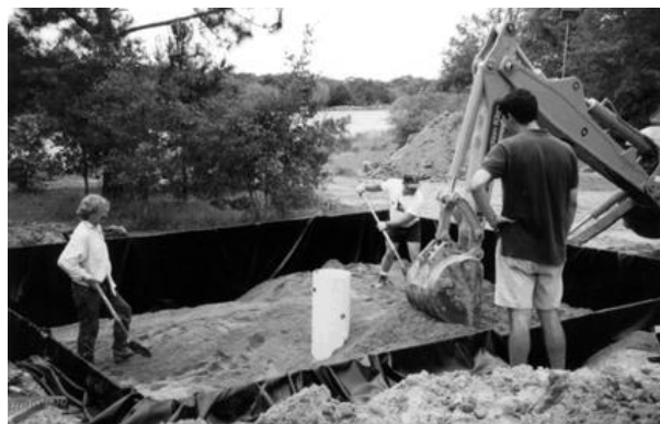
Jim Bonner (far left) supervises construction of a sand filter. This work replaced an on-site wastewater system at his College Station home. Steven Murdock (in back) of Infiltrator helped install the system, while Steve Gonzales of the Brazos County Health Department observed the installation.
