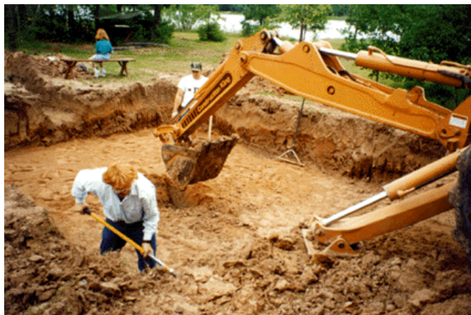
Jim Bonner (with shovel) helps excavate the area where his on-site wastewater system will be installed.
