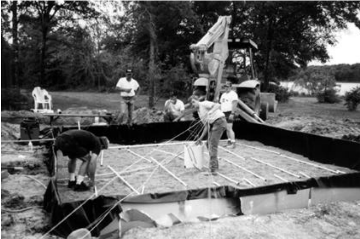
This pressure distribution manifold (above) will evenly distribute wastewater onto the sand filter.
