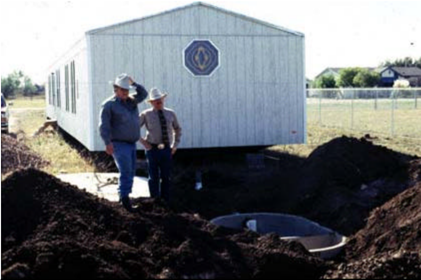
Topper Rawlings and Mike Loving look at this septic tank that was installed to service a mobile home at Grape Creek.
