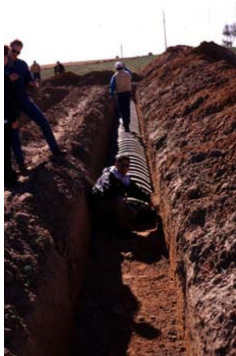
This photo shows a leaching chamber being installed. Leaching chambers are attractive in many areas of Texas because they reduce the amount of land that needs to be dedicated for a drainfield.
