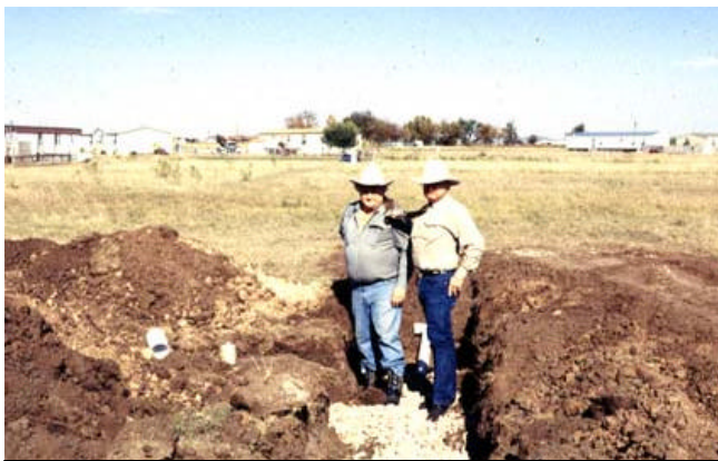
Topper Rawlings and Mike Loving check on the progress of this on-site system being installed near Grape Creek. In this case, a large amount of excavation was required.
