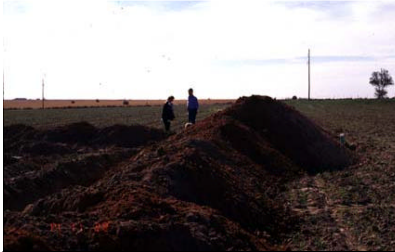
This photo shows piles of dirt that were excavated to install an on-site wastewater system.
