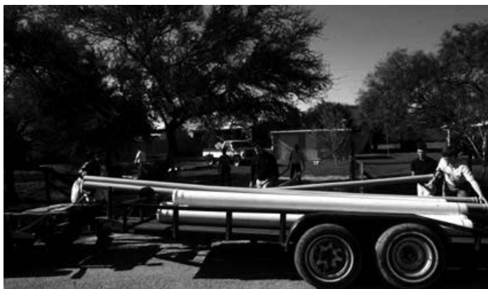
STEP efforts will replace failing septic tanks with this new collection system.
