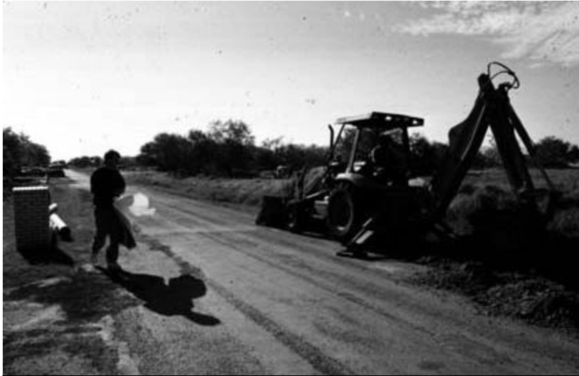
A major part of this project involved burying existing septic tanks and excavating areas for a new collection and distribution system.
