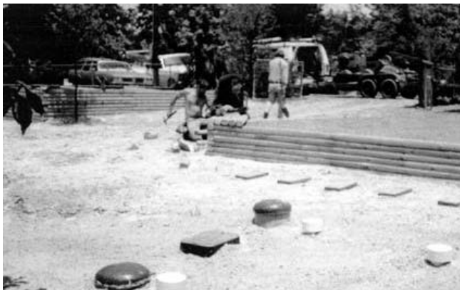
In this photo, an existing septic tank and drainfield is being replaced by an aerobic treatment unit. Variations of aerobic units can provide better treatment, especially in sites like this on small lots.
