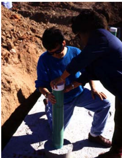
Amy Sanchez and Ric Jensen work to open this inspection port on a newly installed septic tank.
