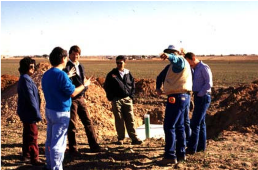
Officials from the Lubbock Region of the TNRCC and the Lubbock City County Health Department discuss the installation of this leaching chamber. Ric Jensen of TWRI has his back to the camera and is wearing a blue sweater. Amy Sanchez of the TNRCC Lubbock office is at the far left.
