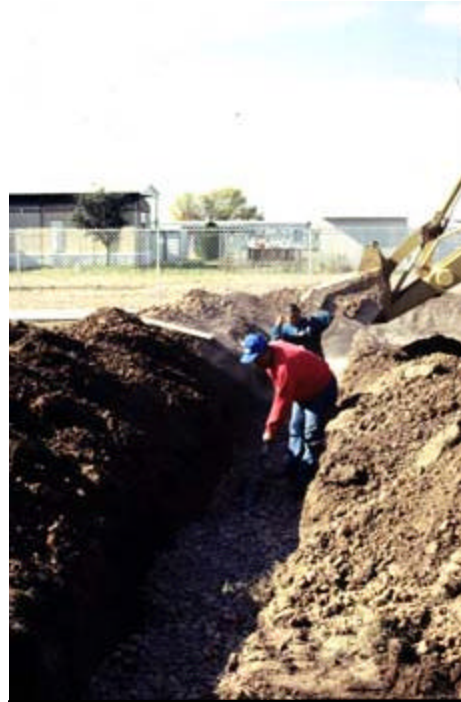
This photo shows the amount of gravel that has to be imported to install on-site systems. The cost of gravel is a major factor that affects overall system expenses.
