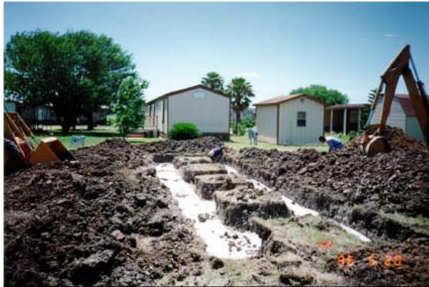
This drainfield was installed to serve a mobile home near Indian Lake in the Lower Rio Grande Valley. In this case the drainline was covered with a geotextile fabric.
