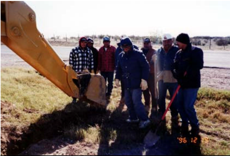
Volunteers and community leaders from Pueblo Nuevo turn the first shovel of dirt to replace failing septic tanks with collector and service lines that will be connected to a small sewer.
