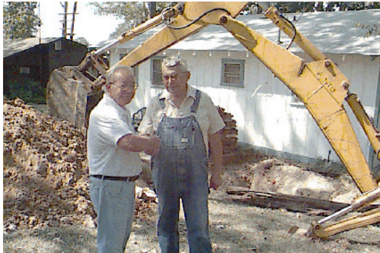
Installer Maurice Short talks with Lee Green about a new cluster system Short installed near Omaha, TX.
