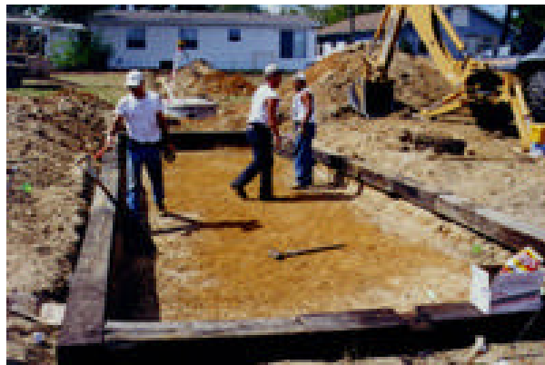
Workers install this constructed wetland at this home in Gregg County as part of the SEP Program.
