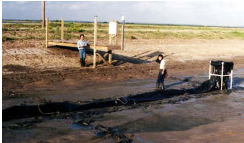
UH graduate students Q. Guo and H. Li install a heat exchange diffuser in a thermal refuge at an aquaculture facility in Palacios, TX.
