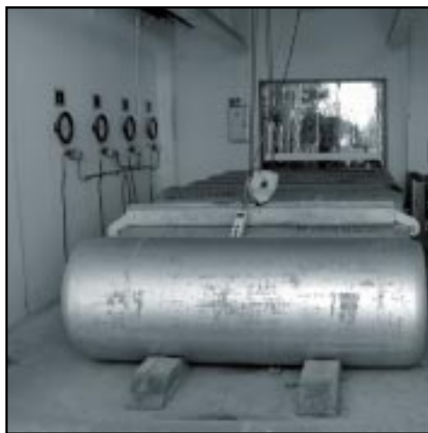
One-ton gas cylinders contain chlorine used to disinfect drinking water poses a respiratory and skin blister hazard.
