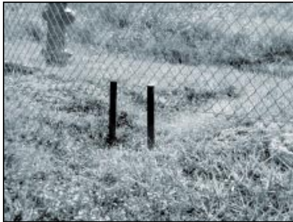
A washout under a perimeter fence could present a security hazard at a water or wastewater treatment plant.
