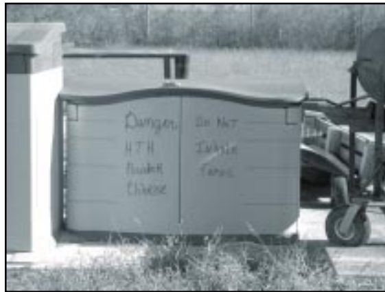
Chemicals used in water treatment should be kept in a secure area.
