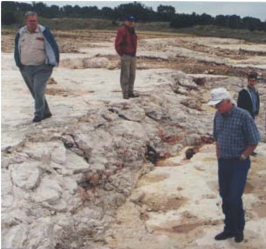
Fernando Garza and Allan Colwick of the NRCS, Jim Blair of SARA, and Jaime Villena of the TNRCC (shown here from left to right) look at erosion damage resulting from the 1998 floods at a small dam on Salado Creek.
