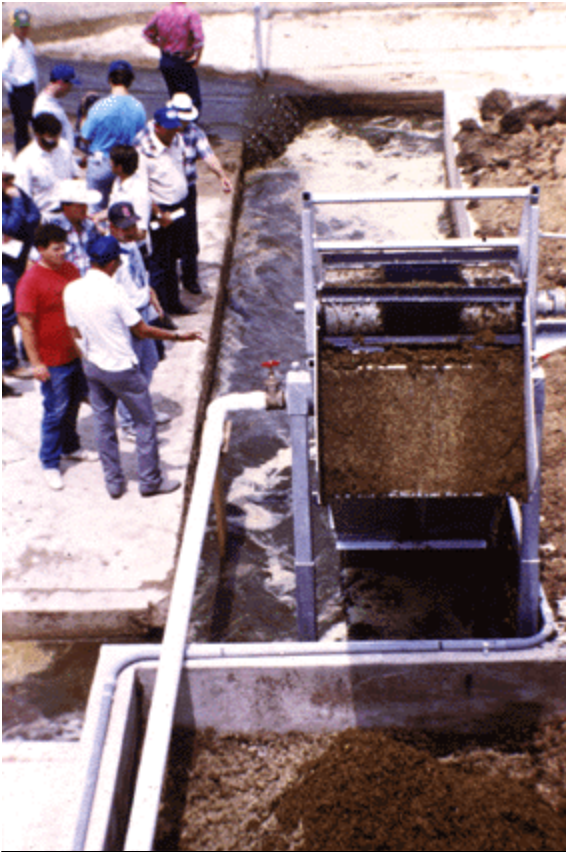
Participants in a field day at the Lake Fork Creek HUA Project observe how this solids separator operates. The separator improves water quality from dairy wastes and small municipal wastewater systems.
