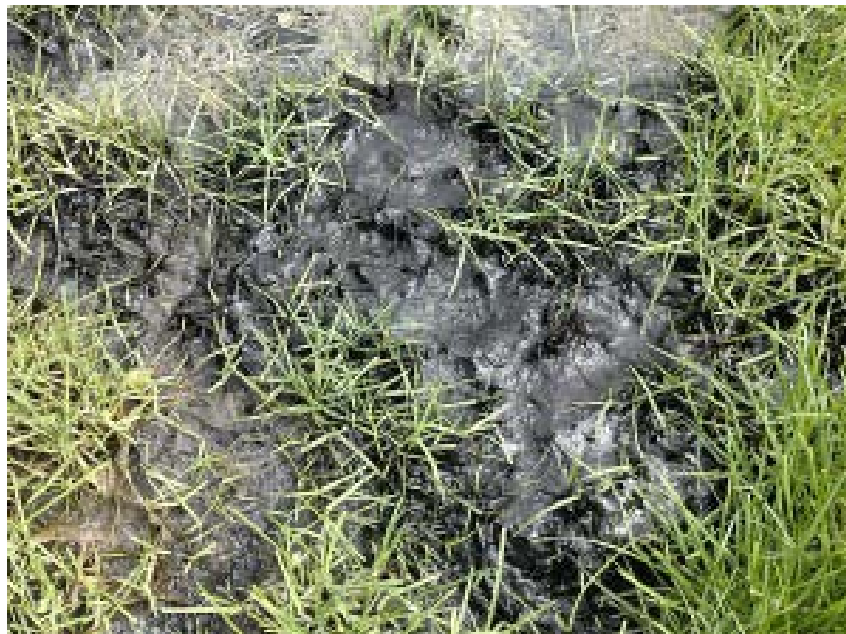
Figure 5.5. Surfacing effluent is a symptom of septic system failure that can be caused by several factors such as poor soil suitability, age of the system, or overloading. Photo courtesy of FirstCallSeptic.com.
