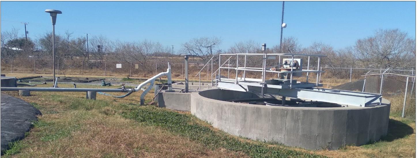
WWTF clarifier. Photo courtesy of NRA.
