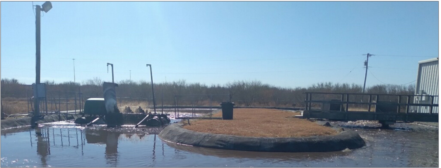
WWTF raceway. Photo courtesy of NRA.
